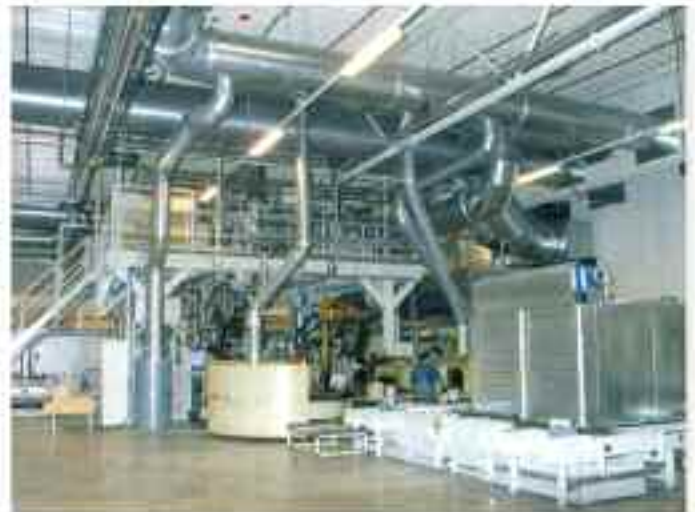
Automatic prepolymer production unit
